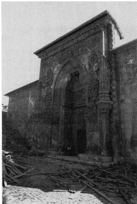
Figure 4.8. Sivas, Divrigi, Ulu Cami, current roof repairs. Some of the tumbled timbers show signs of 20th century machine-cutting. Others are adzed beams from the 13th century. (P. I. Kuniholm, ADP)
